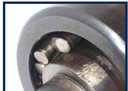
Catastrophic Failure of the Bearing
